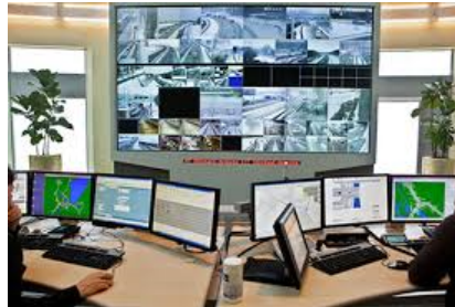
Traffic control centre
